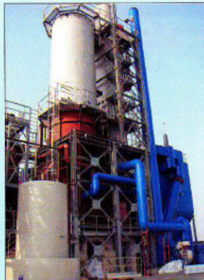
Classen biomass-fired heating plant in combination with a ORC-cycle based de-centralized power station
